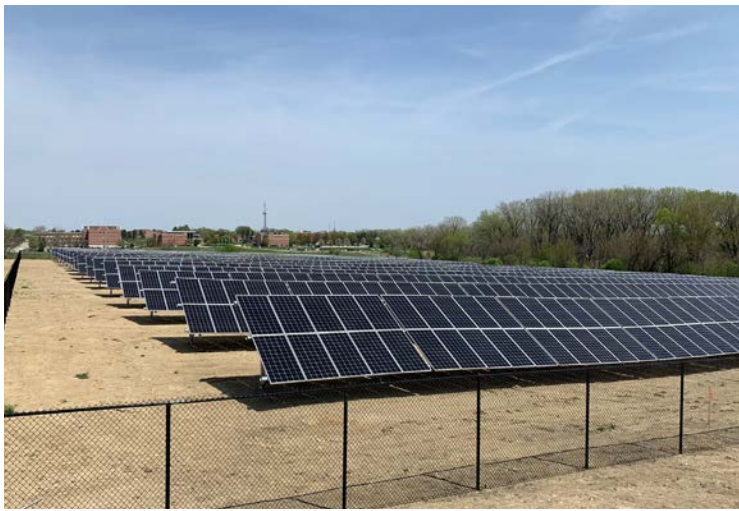
Solar Array, Lewis University
